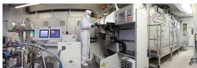
Battery pilot plant in CEA Liten headquarters, Grenoble, France
